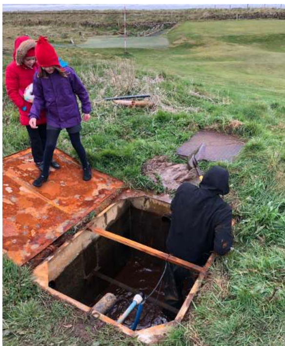
The Team sorting out the blockages
