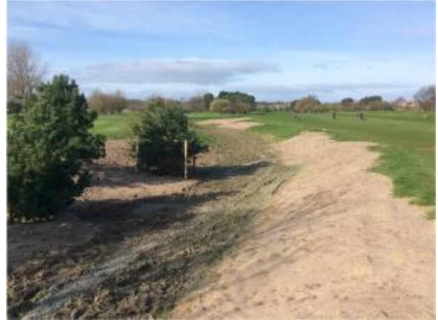
Figure 12: The work to the swale on the 8 th has been mostly completed and the focus now is on finishing off topsoil integration to the base and regaining grass cover through seeding.
